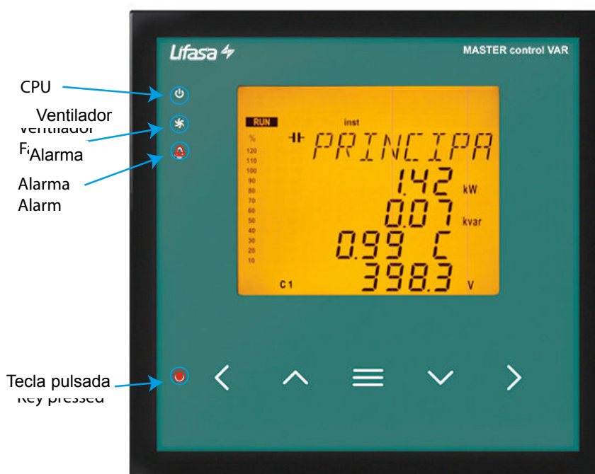
Figura 15:Indicadores LED del Controller MASTER control VAR.
